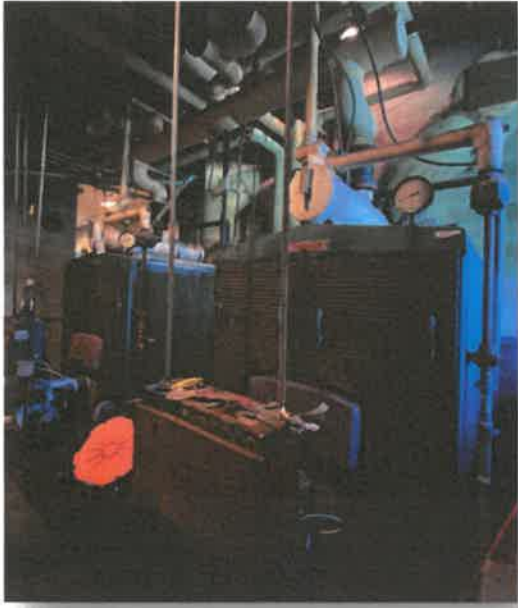
Oil fired boilers at High School.
